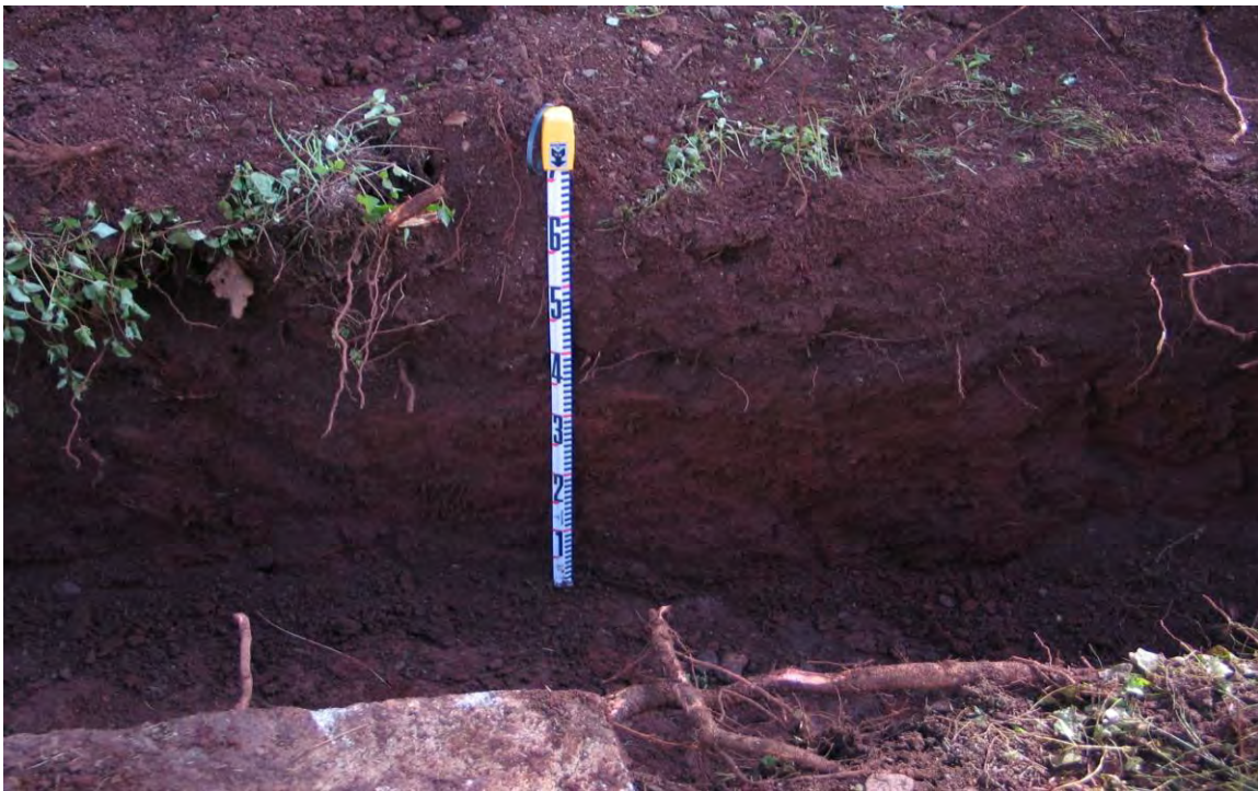
Figure 20: The electrical conduit trench, south of the sidewalk. Note the two distinct layers—the dark reddish-brown atop the dusky, red layer.
