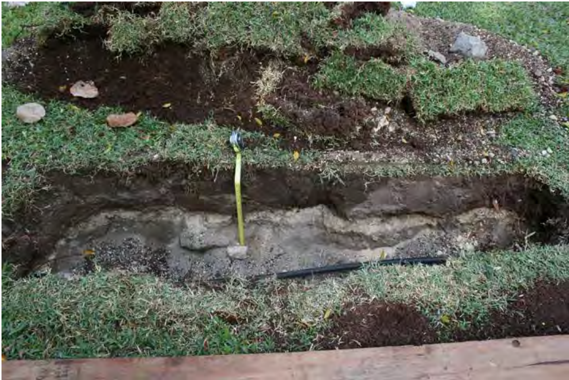
Figure 29: Cable for Video System at Fort DeRussy
