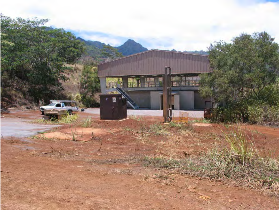
Figure 11: Shoot House, Under Construction. Viewed to the north, from main Range road. Most of the UAC is behind and to the left of this point.
