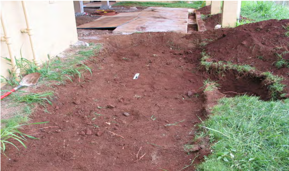
Figure 18: AC unit pad foundation The dry well is on the right. This view is to the north.
