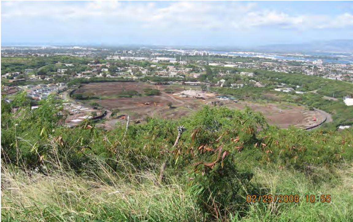
Figure 16: Start of Construction of New Housing at AMR, in 2008. Ground cleared in North half of Crater.
