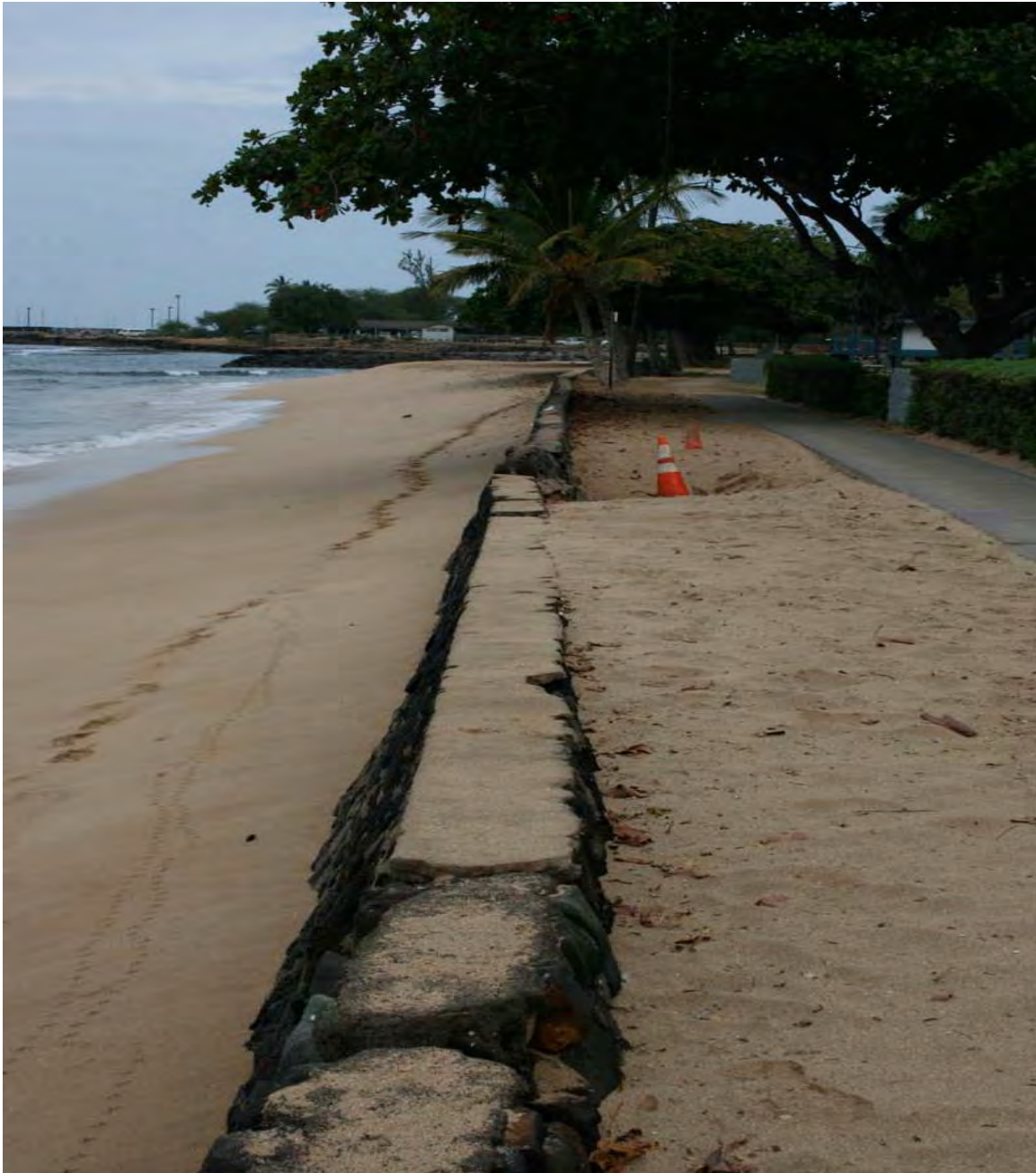
Figure 28: Damaged Section of Existing Sea Wall at PAR. The cones indicate area where erosion at high tide is flushing sand seaward through the damaged sea wall.
